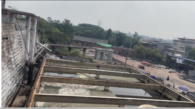
卤水澄清池中残留盐泥
